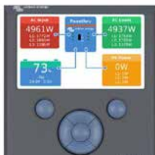
Color Control GX, showing a PV application
